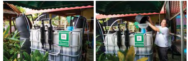
The 11 th SUZDEE system installation station in Nan Province
