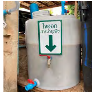
New generation system at Nan Municipality Office
